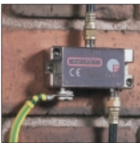
ESP CATV/F installed in a basement or garage near where the coaxial cable enters the building
