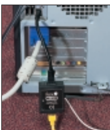
ESP LN installed on the network connection to a PC. Note the black earth lead connection to the chassis of the PC.
