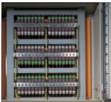
Three rows of protectors, inside a control cabinet, each installed on a CME 16 combined mounting and earthing kit.
